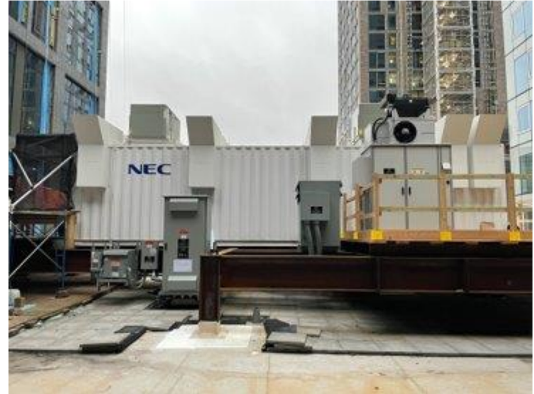
Barclays Center NWS Battery Energy Storage System
