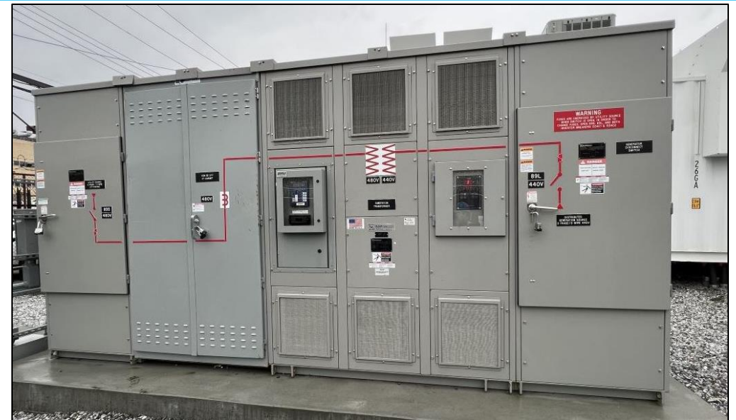
Battery Energy Storage System in Woodside, Queens
