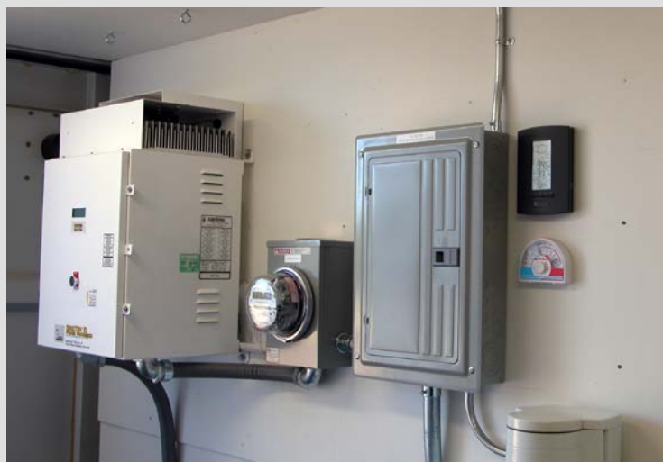
Electrical Equipment – Image Credit NREL Image Gallery #13326
