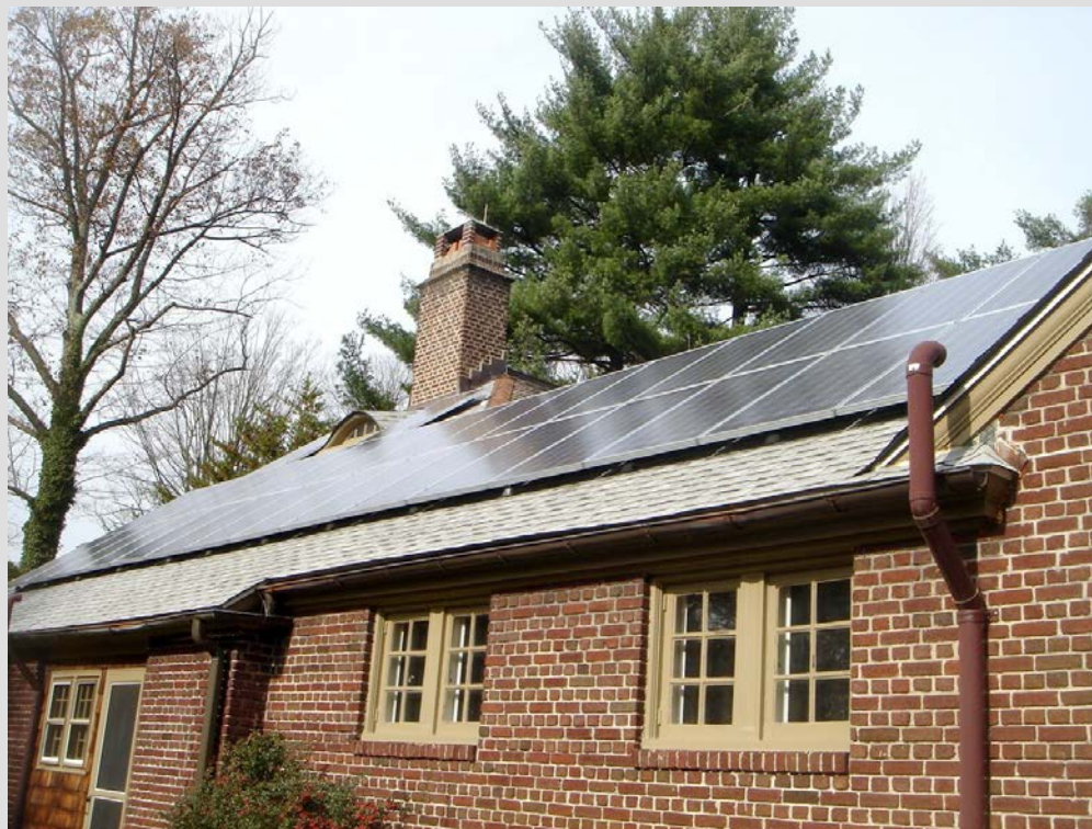
Roof Mounted Solar Array – Image Credit NREL Image Gallery #18067
