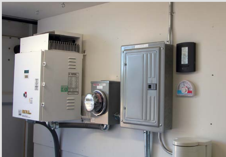
Electrical Equipment – Image Credit NREL Image Gallery #13326
