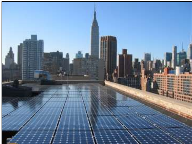
Kips Bay Tower in Manhattan: 20-story condominium building. 54.28 kilowatt solar system provides 57,000 kWh per year.
