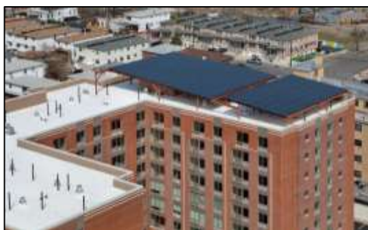
Dumont Green in East New York: 8-story, 176-unit, low-income rental building. 80.5 kilowatt solar system provides power to cover 80 percent of the laundry facilities, elevators, common areas, and security systems.
