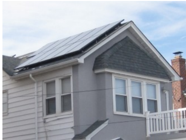
Photo Source: EmPower Solar
